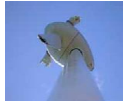
Wind turbine No. 6
