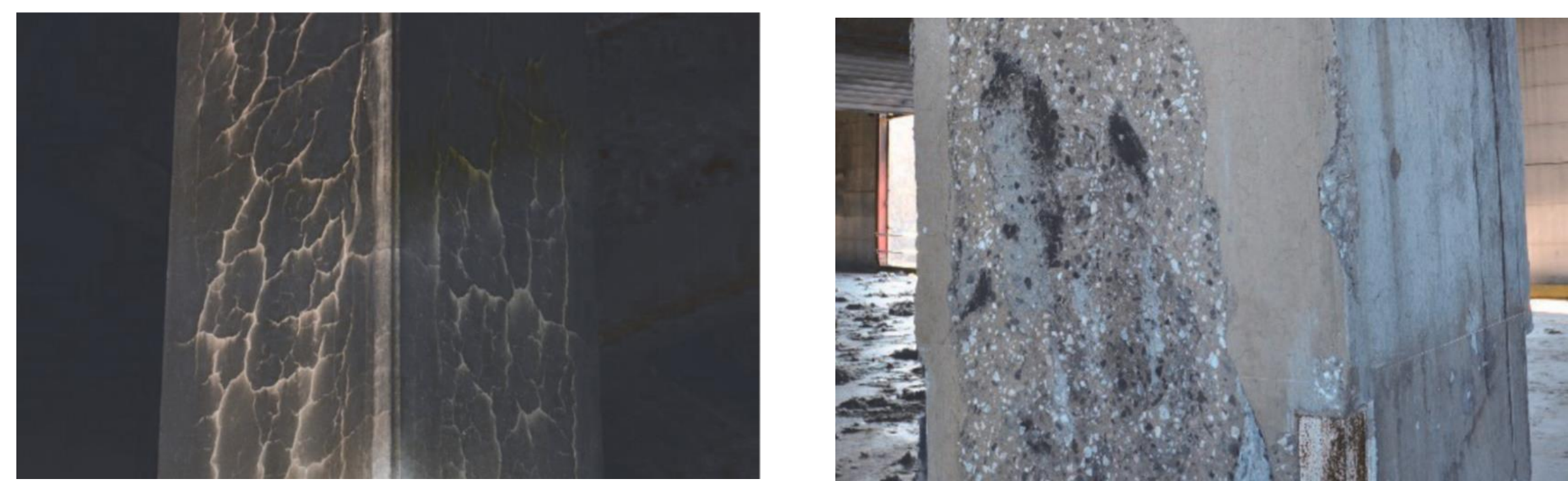
Fig. 2 Visual deterioration of concrete member after fire 1)
